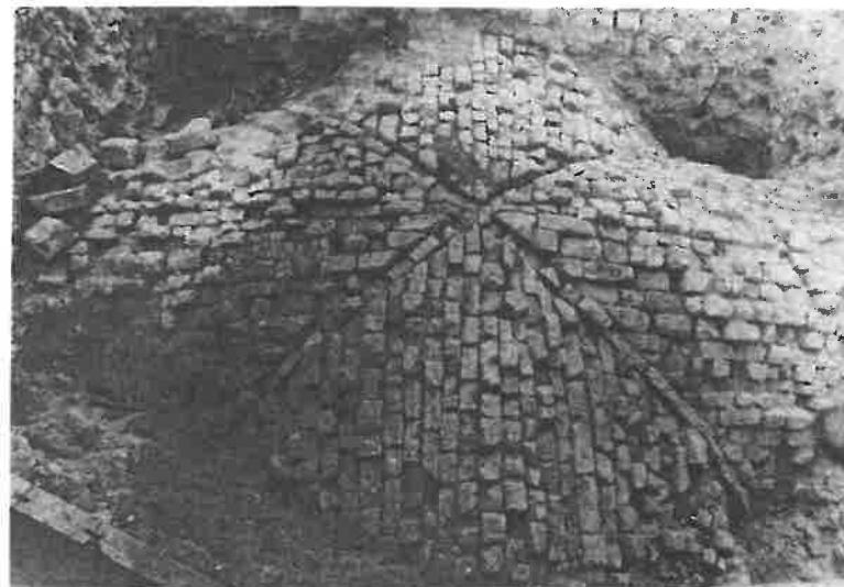
Fig. 5.7. Jerusalem, Holy Sepulchre, extrados of transept vault during repair, showing rib stems between vault compartments. Photo: Virgilio Corbo.
