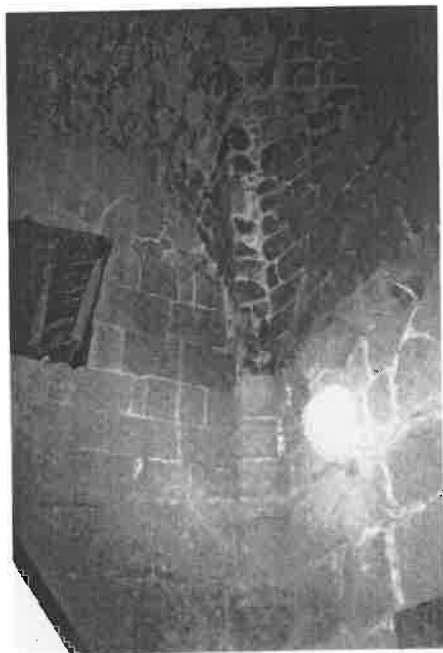
Fig. 5.4. Acre, Compound of the Knights of St. John, vault of latrine, showing springer and exposed arris where rib has fallen, end of twelfth century. Photo: author.
